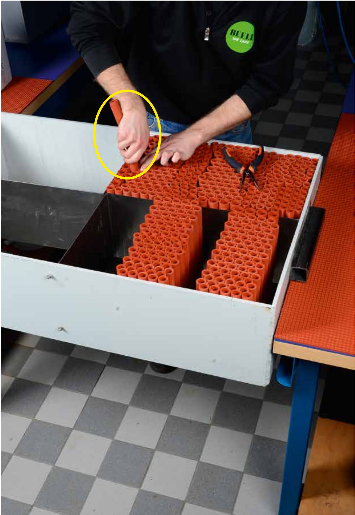
Single filler sleeves are then used to fill the remaining smaller openings.
