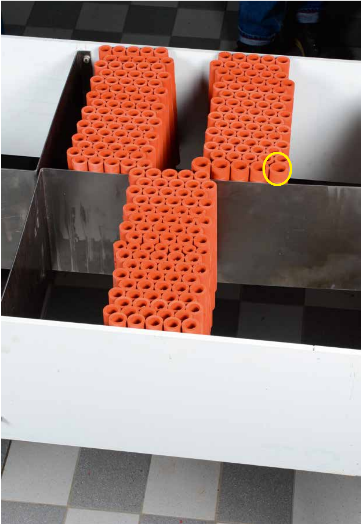
Another set of filler sleeves is inserted. In this case a set of NOFIRNO sleeves 27/19 is used for a good fit for insertion.
