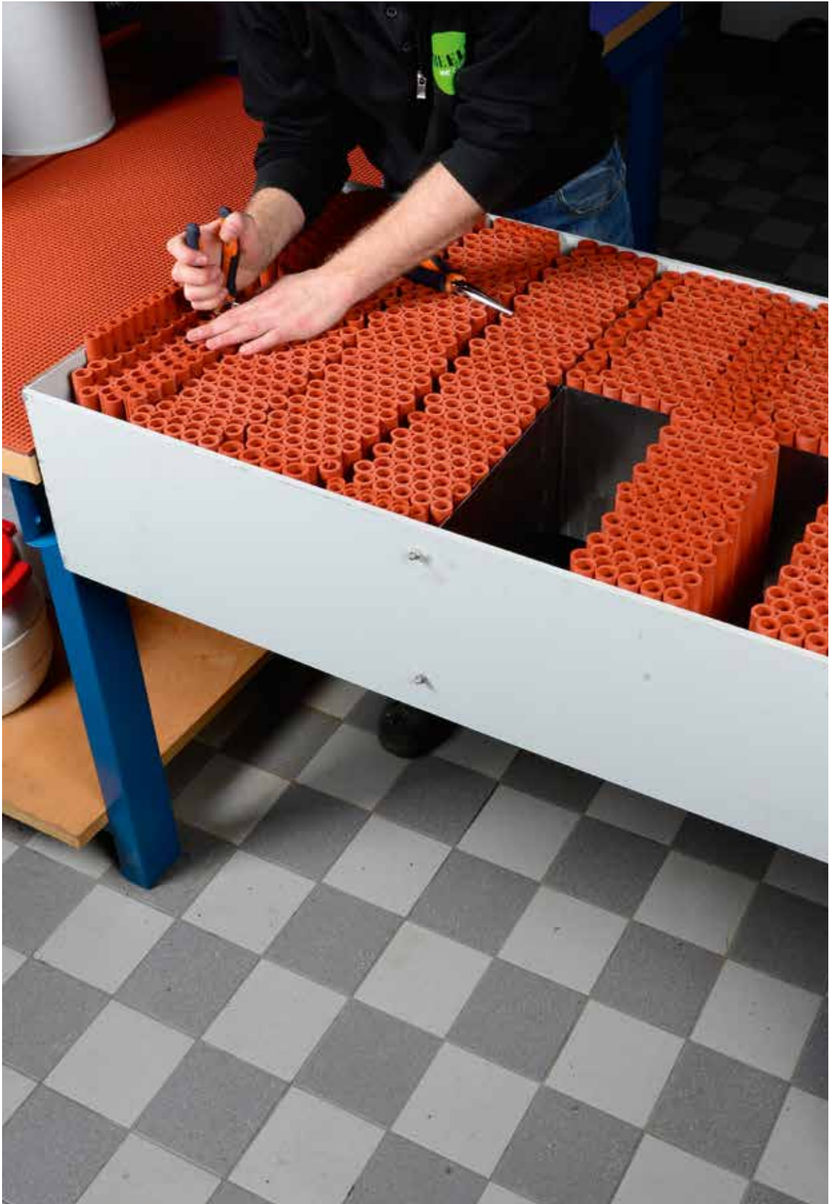
Insertion of more filler sleeves in all smaller openings in the set of fillers to obtain the sufficient clamping forces inside the sections.
